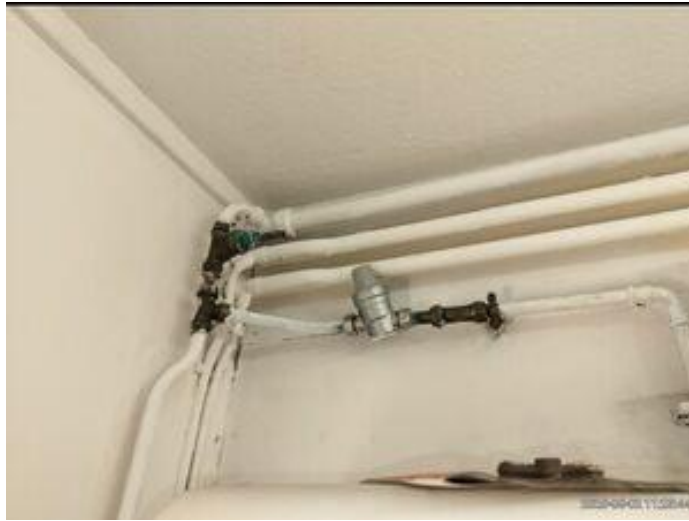
PRV on MCWS spur to LVPOU 1
