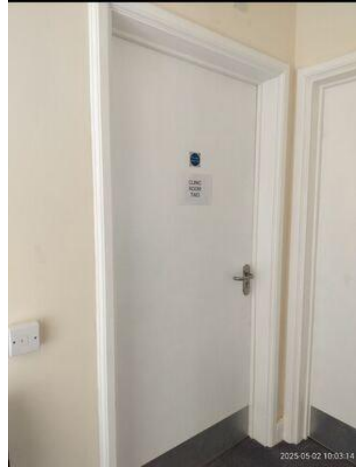
No access to clinic room two however believed to have no water (As traced in loft above also)
