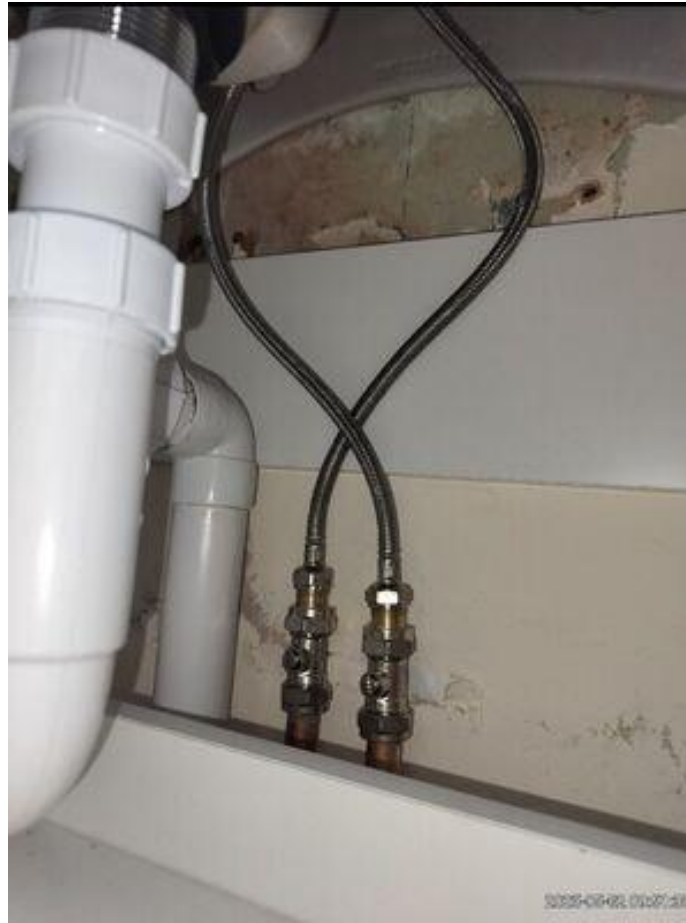
Example of flexible hoses on site
