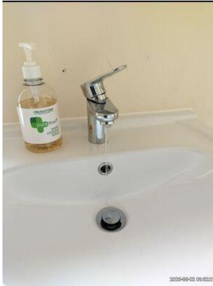
Poor flow from TCWS outlet
