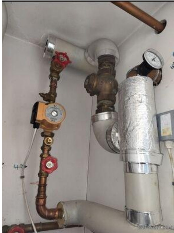
Single check valve on HWS outlet
