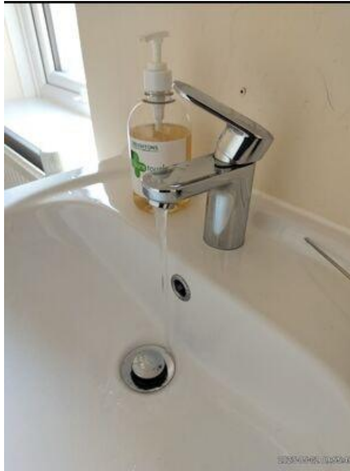
Poor flow from HWS outlet
