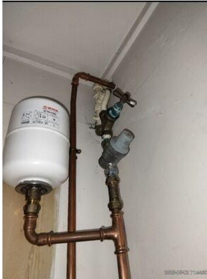
PRV on MCWS spur to HVPOU 1
