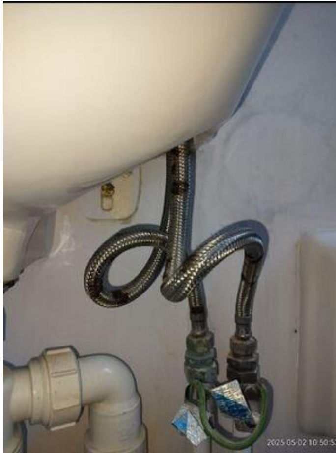
Flexible hoses in poor condition - rusty
