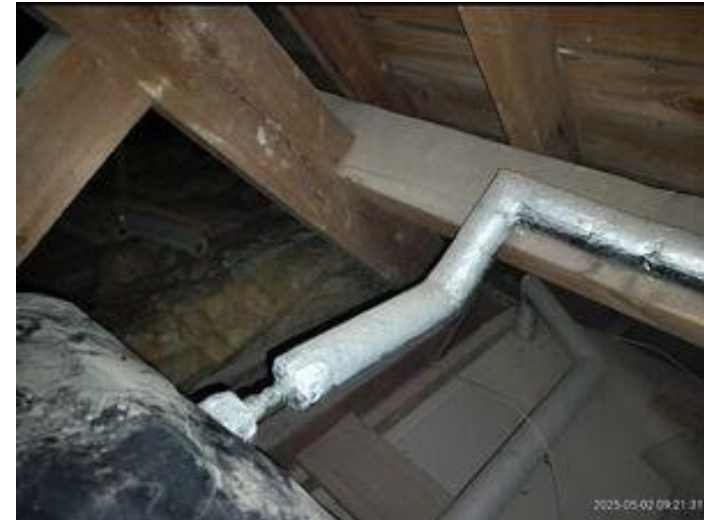
Spur to F&E tank requires adequate backflow protection (double check valve)
