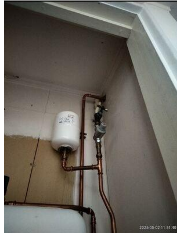
Local isolation to dead end
