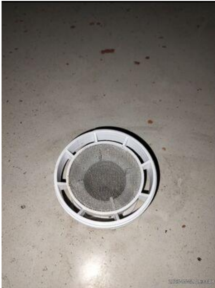
CWST 2 - External - Screened breather fit to the lid is in good condition
