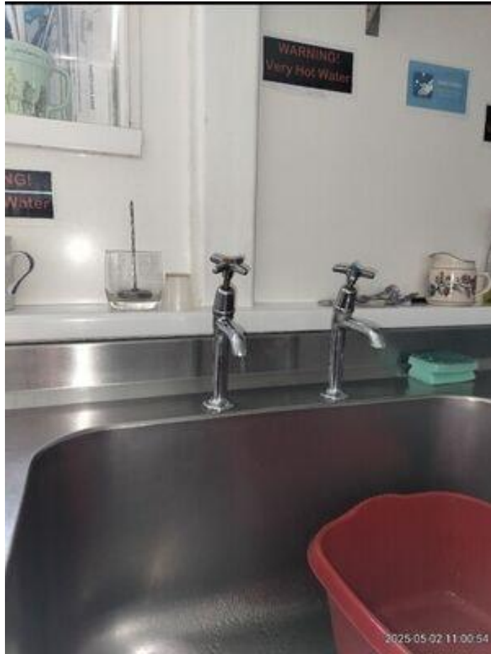
HWS outlet is currently a dead leg - When tap is turned on no water flows
