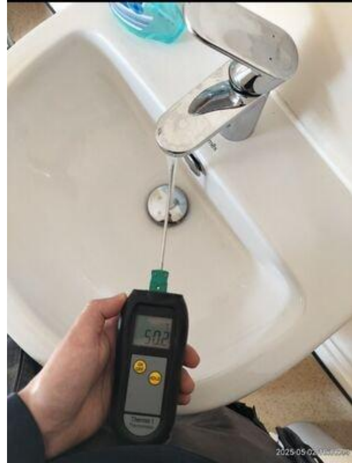
Accessible toilet fit without a TMV at the basin- Currently there is a risk of scalding
