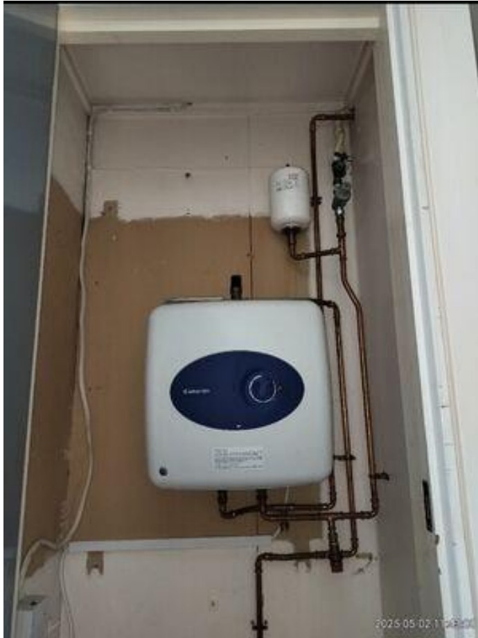
Current PV requires replacing with a 5 litre PV due to the HVPOU size (30L)
