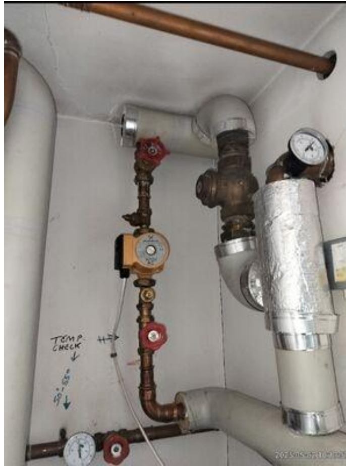
Pump on HWS to site
