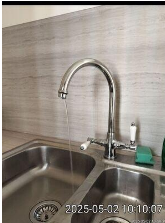
Poor flow from HWS outlet restricted accurate temperature
