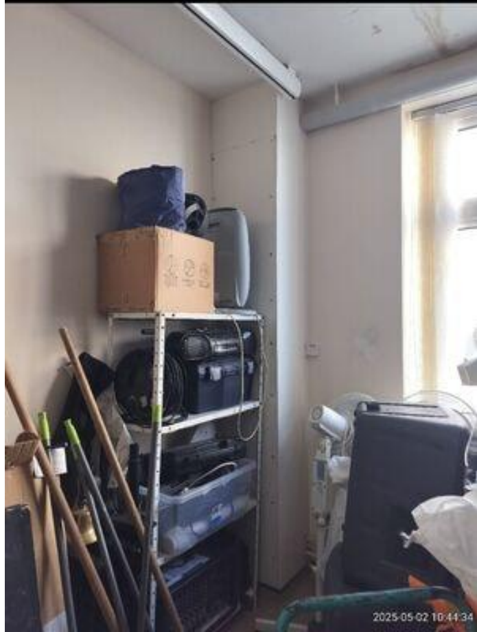
Unable to open boxing where pipework drops/rises due to stuff in the way/shelving
