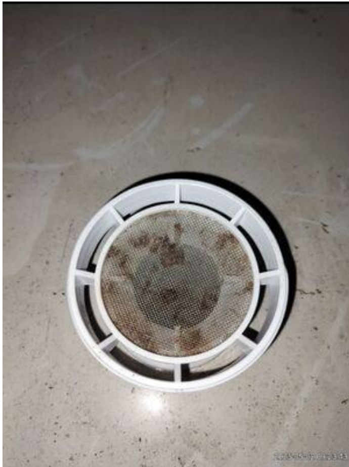
CWST 1 - External - Screened breather fit to the lid is corroded - Recommend replacing
