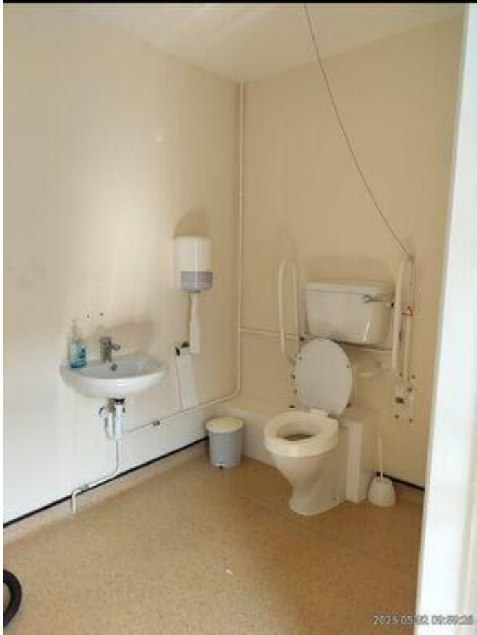
Accessible toilet fit without a TMV at the basin- Currently there is a risk of scalding
