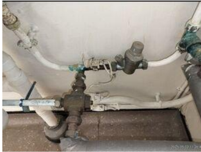
PRV on MCWS spur to basins X2
