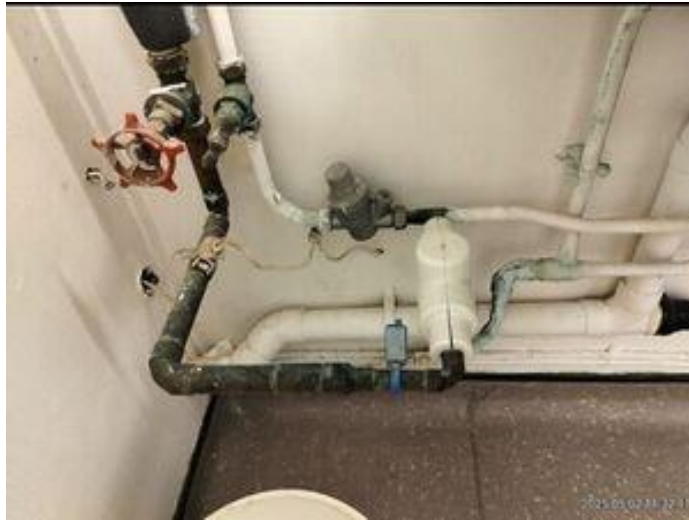
PRV on MCWS spur to basins X2
